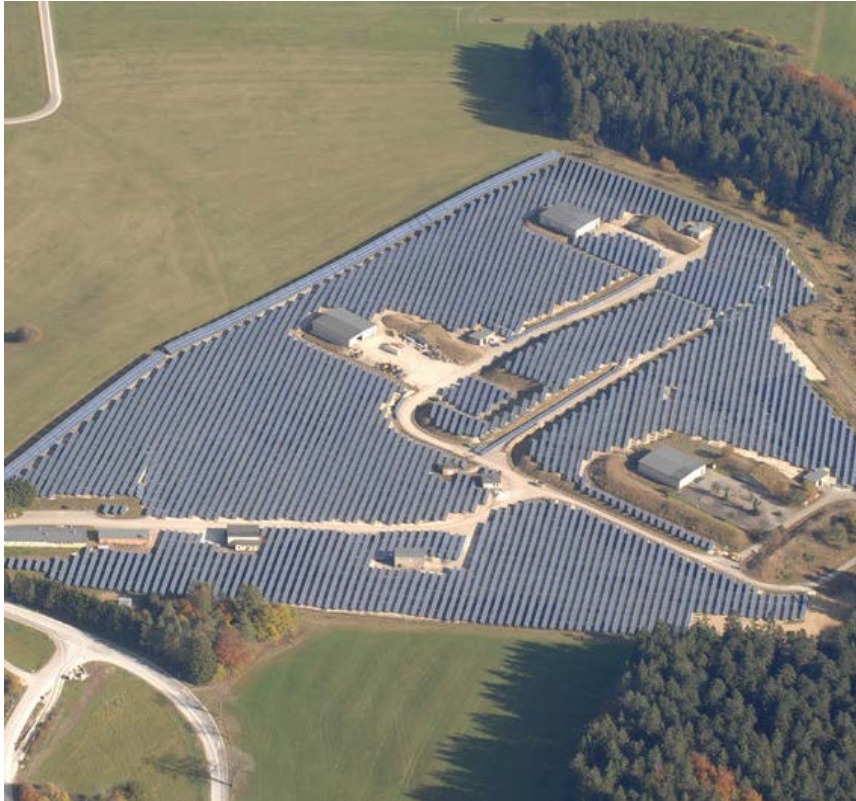
5 MW PV Power Plant "Dürbheim"
